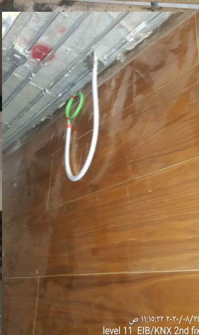
ص 1:30:9 2020/08/17 electrical rooms level 17 for BF Fixtures
