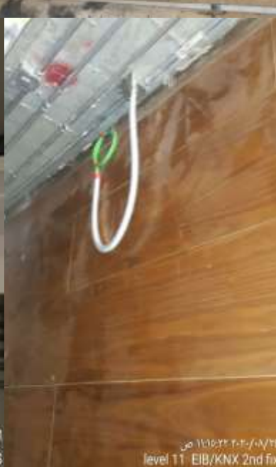
electrical rooms level 17 for BF Fixtures
